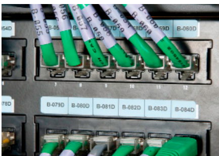
Patch Panel Labels
