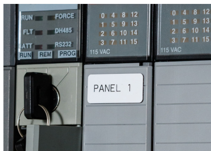
Control Panel Labels
